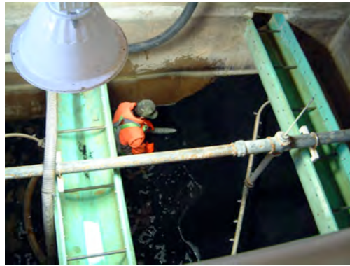
GAC-Capped Sand Filter at Bloomington, IL
