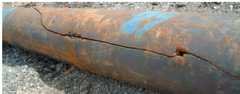
Longitudinal Break through Two Distinct Corrosion Points
