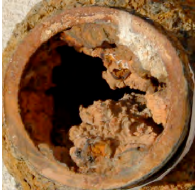
Severely Encrusted 2" Pipes
